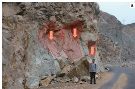
Fig. 6 Rock mass with significantly open fissures
